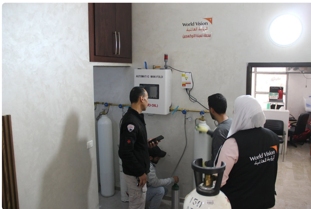
A new oxygen refilling station at a Trauma Stabilisation Point. © World Vision
